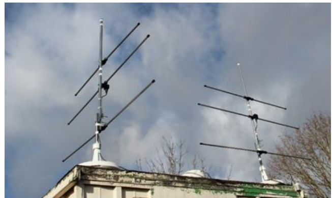
Figure 8 – Two FM Yagi antennas on the top of the shelter.
